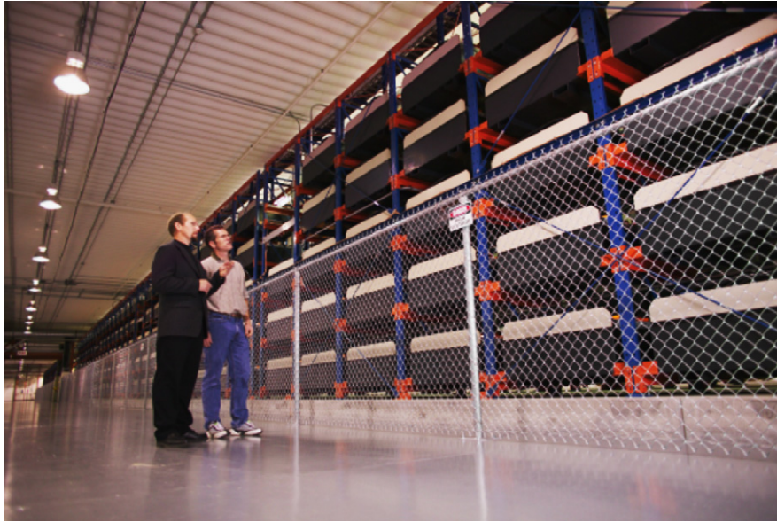
Fig. 1. GVEA battery energy storage system.
